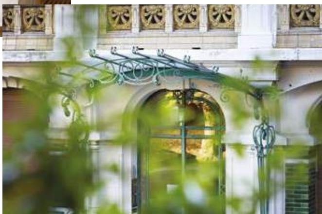
Detail at a former luxury hotel in the spa area
